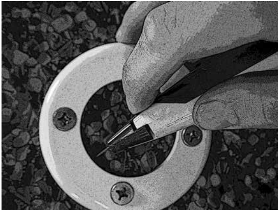
Trim liner from return opening.
