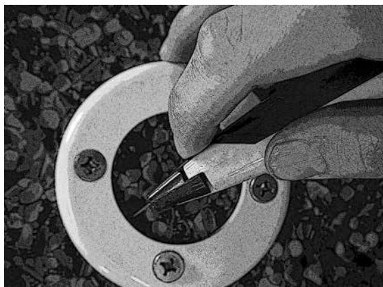
Trim liner from return opening.
