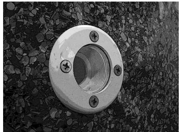
Return faceplate installed.
