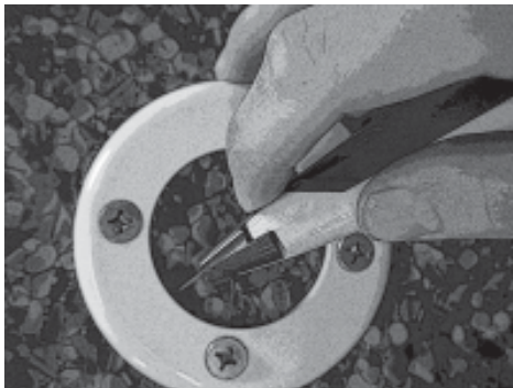
Trim liner from return opening.
