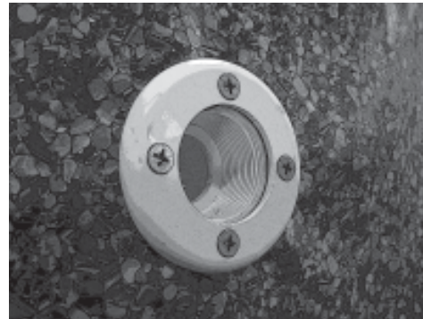
Return faceplate installed.
